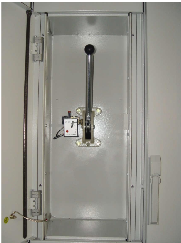
图 6.2 隔离开关闭合时操作杆位置/ Figure 6.2 The position of disconnecter lever closed
